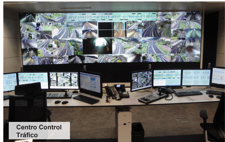
Sala de Control Build Management System
