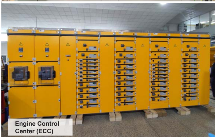
Own electrical panels workshop
